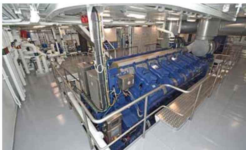
▲ Overall view of the engine room.
