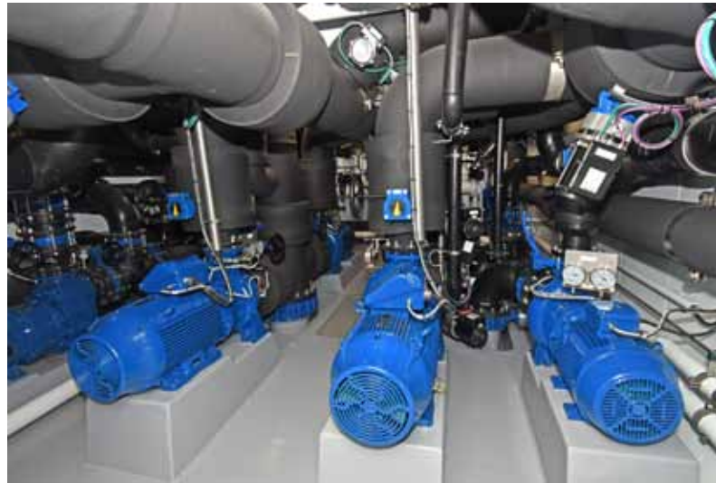
▲ Chilled seawater is circulated through Serene's 11 RSW tanks by 4 x 500m 3 /hr pumps.
