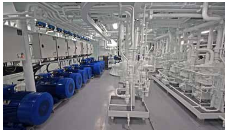
▲ The hydraulic room is arranged across the full beam at main deck level aft.
