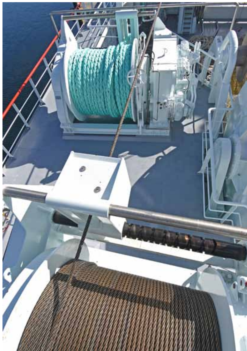
▲ The lifeline winch is mounted on the upper boat deck, aft of the starboard trawl winch.
