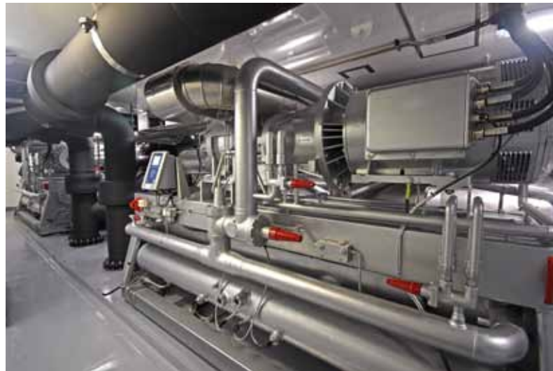
▲ Two ammonia-based refrigeration plants, centrally positioned on the main deck, each deliver 1,450kW of cooling capacity.
