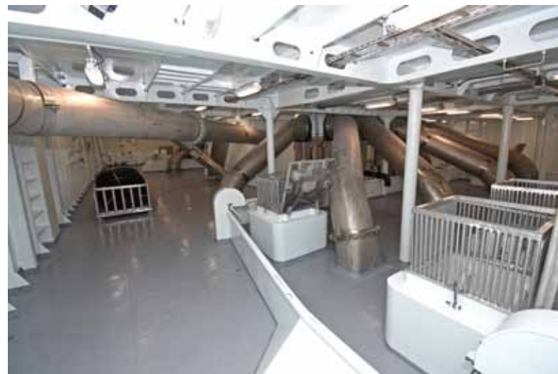
▲ The delivery pipe leads from aft to the dewatering unit, from which fish are delivered to selected RSW tanks.
