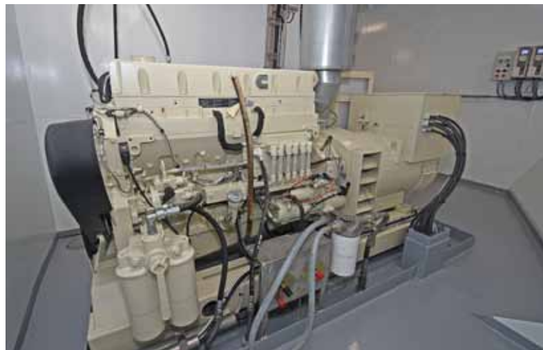
▲ The Cummins QSM11-DM 250kW harbour/emergency genset located forward.
